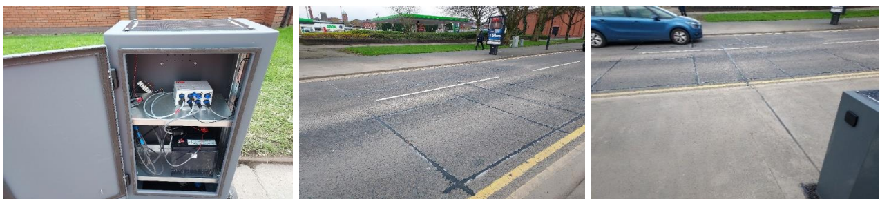
Oldham, A669 Middleton Road, Chadderton: Example of a typical permanent Automatic Traffic Counter (ATC)
